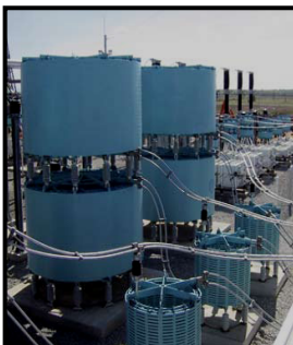
Plinth mounted H.V. Harmonic reactor
