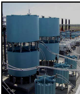
Plinth mounted H.V. Harmonic reactor
