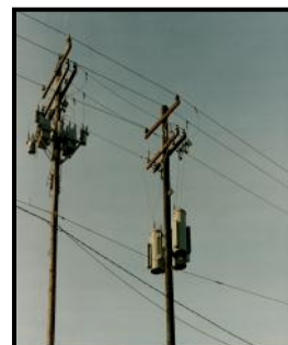
Pole mounted harmonic filter
