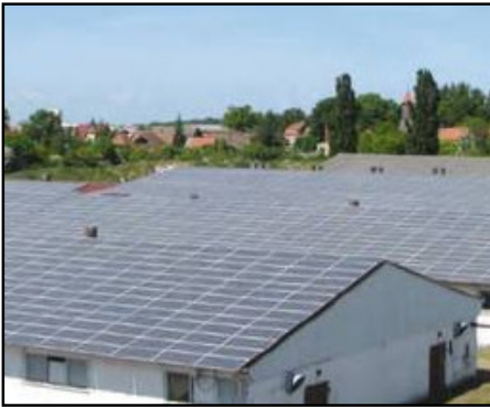
Photovoltaic power plant (DISTRIBUTION/TRANSMISSION)
