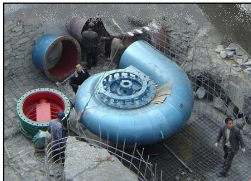
Micro hydroelectric power generation
