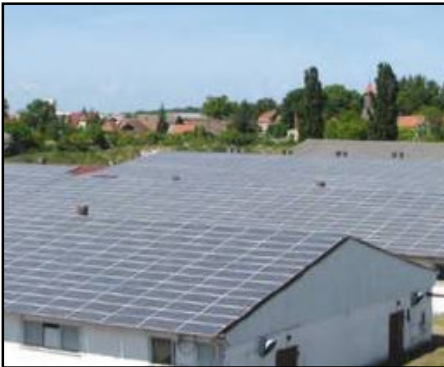
Photovoltaic power plant (DISTRIBUTION/TRANSMISSION)
