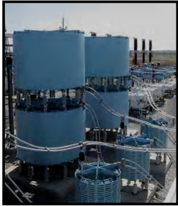
Plinth mounted H.V. Harmonic reactor
