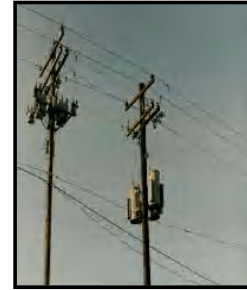
Pole mounted harmonic filter
