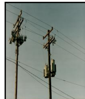
Pole mounted harmonic filter
