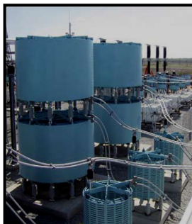
Plinth mounted H.V. Harmonic reactor
