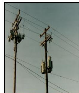
Pole mounted harmonic filter
